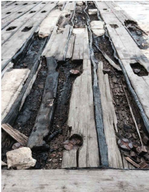
Area of rotted teak on the 01 Level of the ship. This area is Phase 7 on the teak replacement plan.
